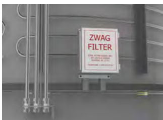
Junction Box on Unit
